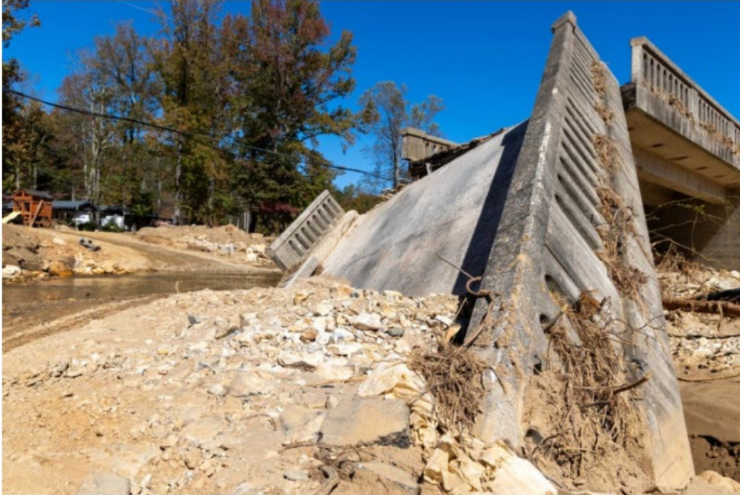
This collapsed bridge in Marion over the North Fork Catawba River was one of about 150 damaged bridges after Helene. (Photo by Travis England/US Army Corps of Engineers)
